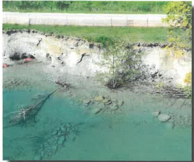
Erosion damage at Bluff Road
